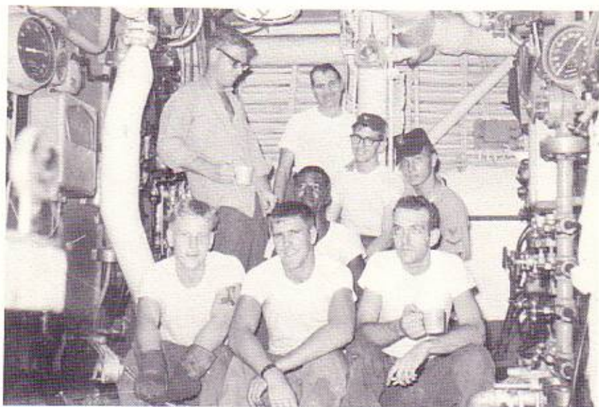
BLACK GANG Forward Fire Room
